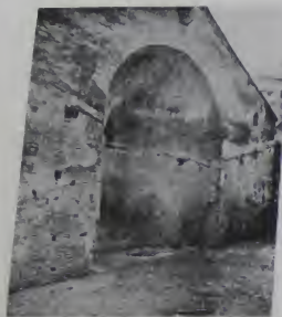
Fig. 154a. S. Maria degli Alessandri (interior, apse wall, and arch from north, 1926 to 1928).
